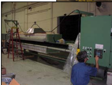
HUMASORB® Treatment Unit for Removal of Toxic Metals from Wastewaters at U.S. Army-Johnston Island
